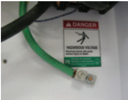
Fig. 7 — A separate, properly sized incoming ground wire is required to protect from electrical shock.
